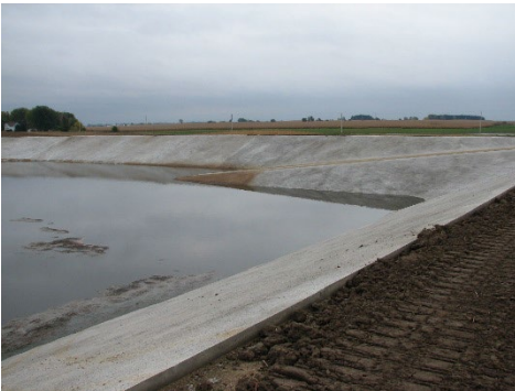
One landowner installed new manure storage system
